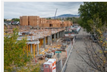
Framing has started for the West Sherwood Apartments (front). Construction on these student housing projects is farthest along at the La Pointe Apartments (rear). Photo by Pete Grady.
