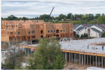
Framing has reached three stories for the La Pointe Apartments (left), while the concrete podium has been poured for the River Edge Apartments. Photo by Pete Grady.
